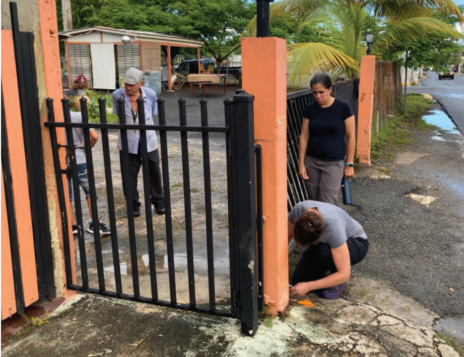
Installing water level loggers at a house on the Caño Martín Peña estuary Photo: Alana Hanson
